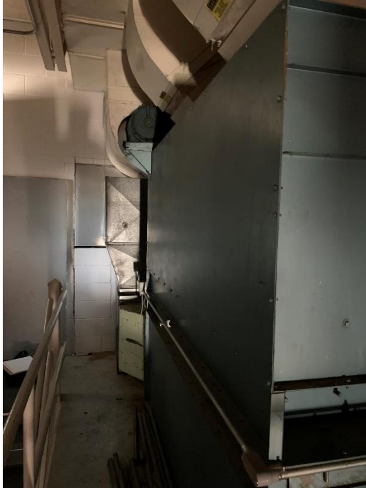
Original Gymnasium Air Handling Unit
