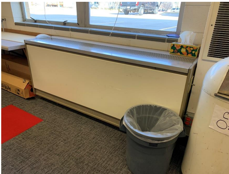
Typical Classroom Unit Ventilator
