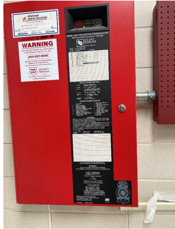
Main Fire Alarm Panel
