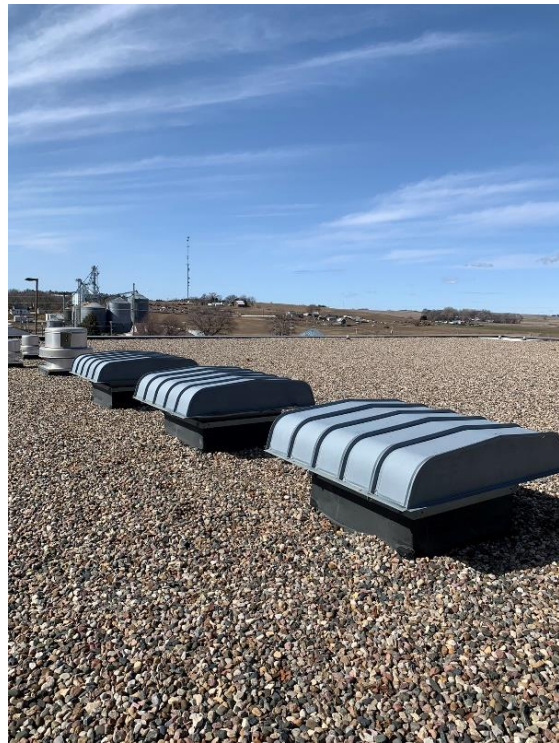
Gymnasium Air Intake Hoods and Exhaust Fan
