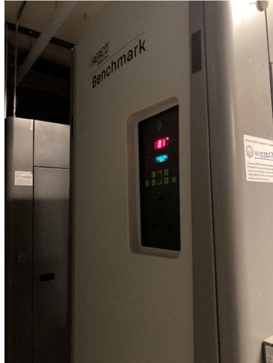
Hot Water Boiler
