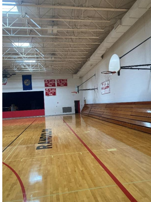
Original Gymnasium Ductwork
