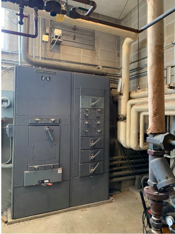
Main Electrical Switchboard
