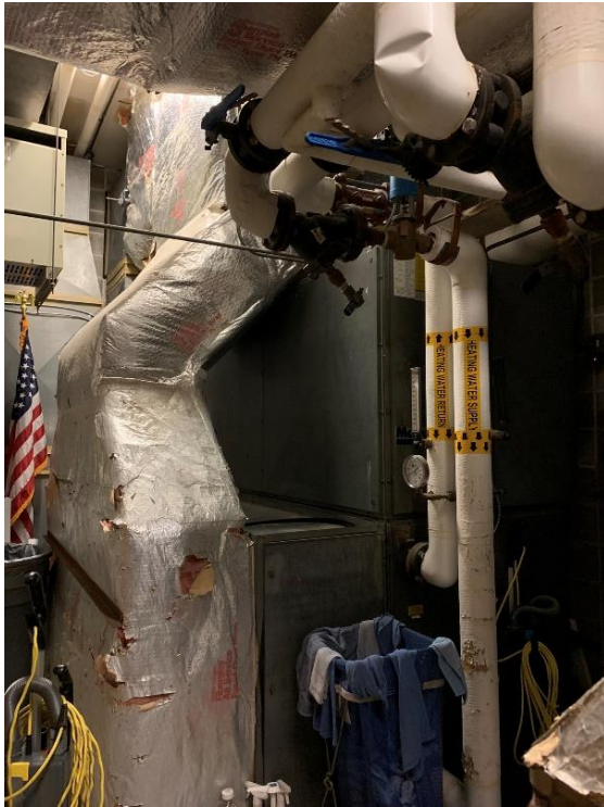
Gymnasium Air Handling Unit
