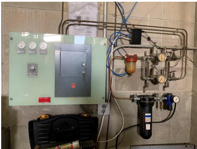
Existing pneumatic temperature controls
