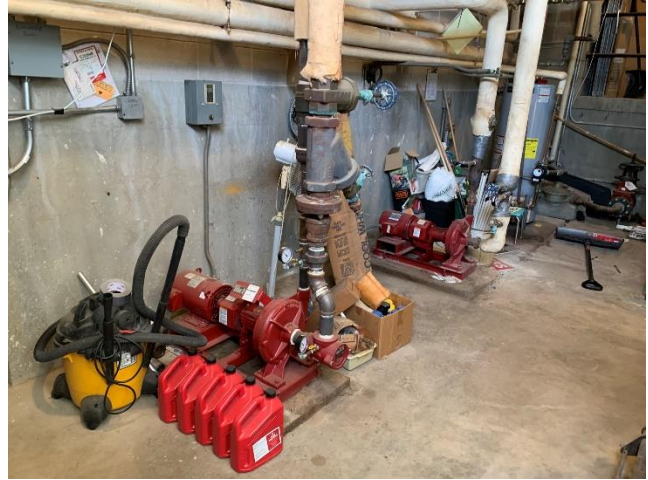
Heating Water Pumps
