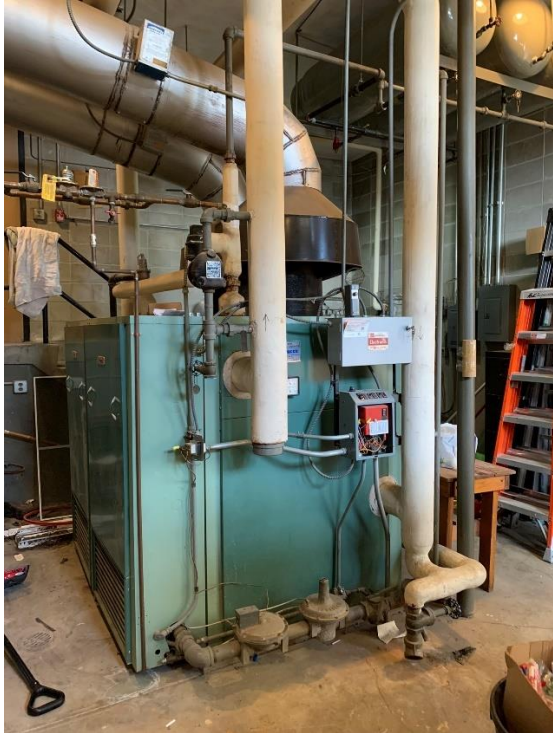
Hot Water Boiler
