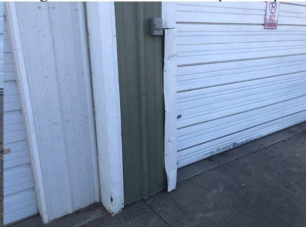
Typical damage at overhead door jambs
