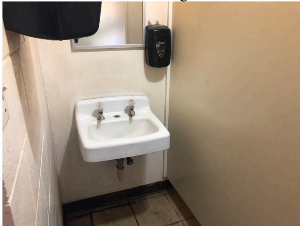
No insulation on lavatory piping to prevent burns, mirror set too high, paper towel dispenser set above reach range.
