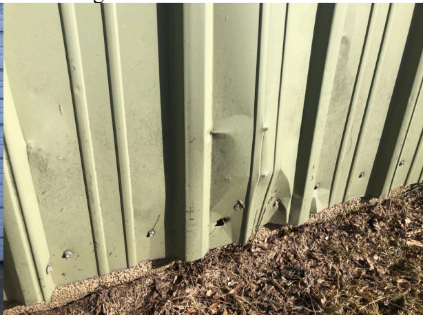
Typical siding damage
