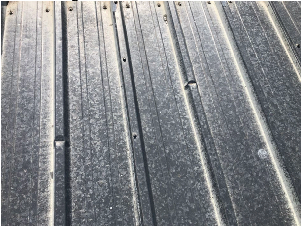
Hail damage upper right and rib damage
