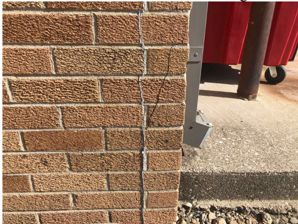
Crack in brick
