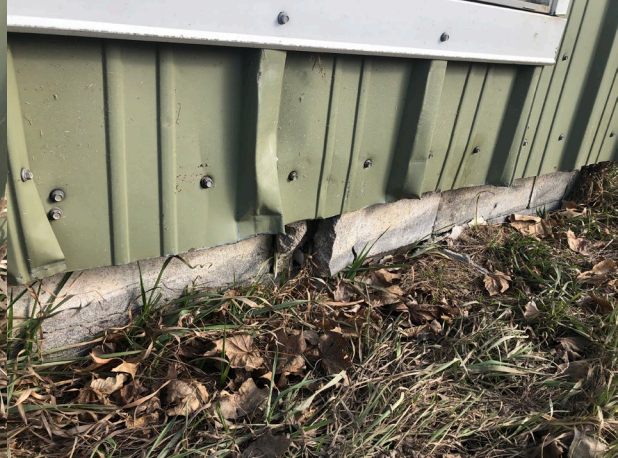
Broken CMU and cracked mortar
