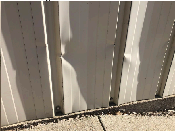
Typical siding damage
