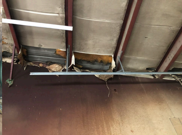
Existing insulation inadequate and damaged
