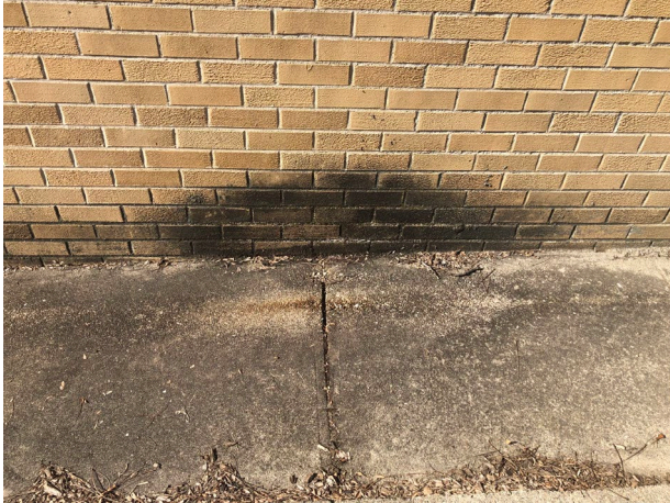
Algae on wall and sidewalk deteriorating under gutter seam that is leaking
