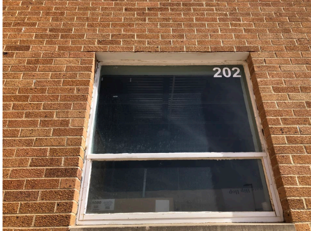
Sealant around window is deteriorating
