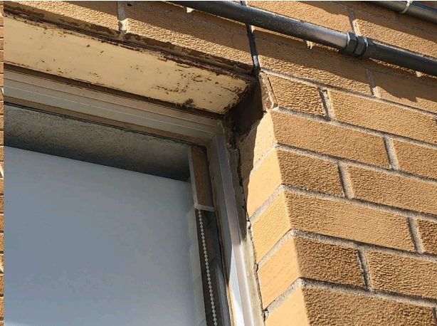
Cracked brick at window head
