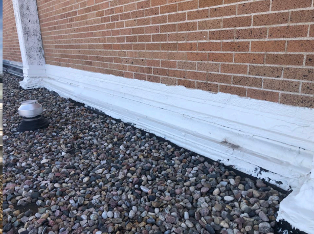
Leaks at the original gymnasium north wall can not be stopped in this fashion. The wall must be sealed and a rain screen added.
