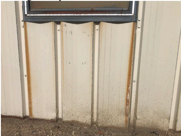
Grade to high panels buried in dirt – rust
