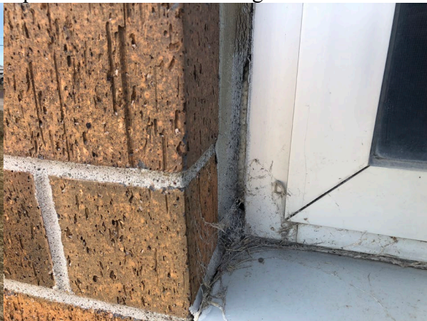
Stress cracks in sealant show that it is losing its flexibility
