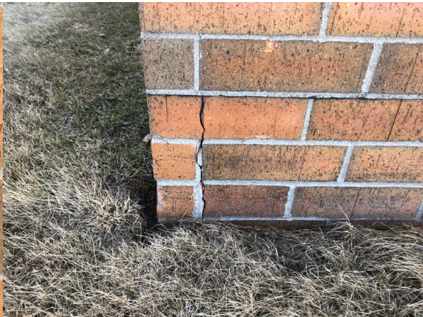
Crack in brick / grade does not slope away
