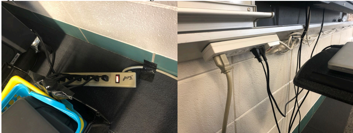
This 6 plug multi-outlet was plugged into.....this 6 plug outlet which was fed by an extension cord. This is a typical problem.
