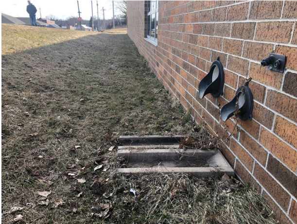
Grade on the east side of the building is running toward the building
