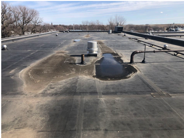
Fully adhered EPDM / standing water should be eliminated
