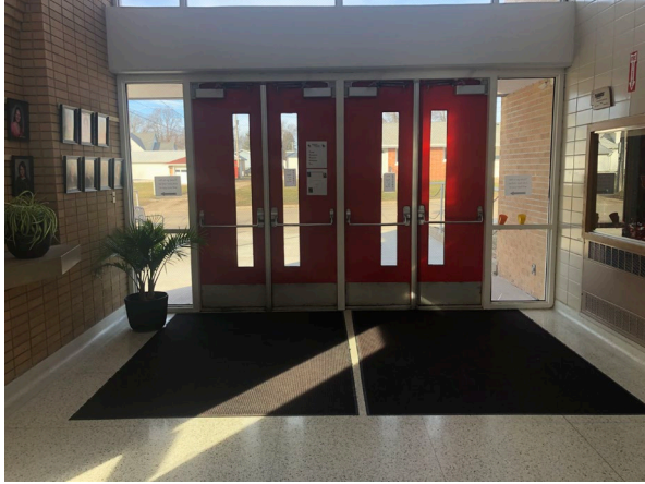
Main entry doors are too narrow to meet ADA
