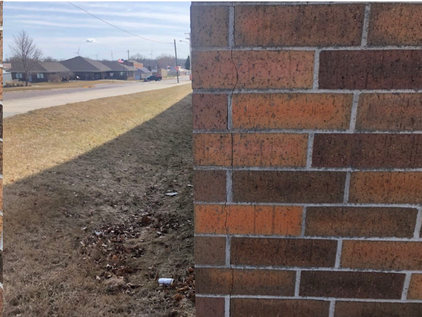
Crack in brick
