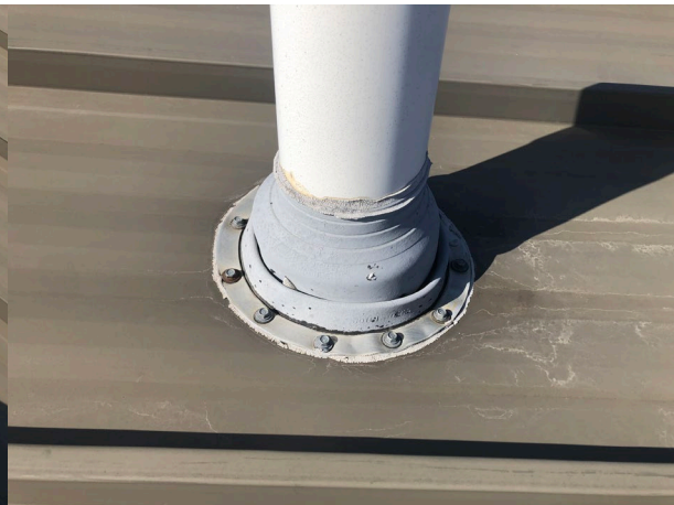
Sealants drying out and starting to crack
