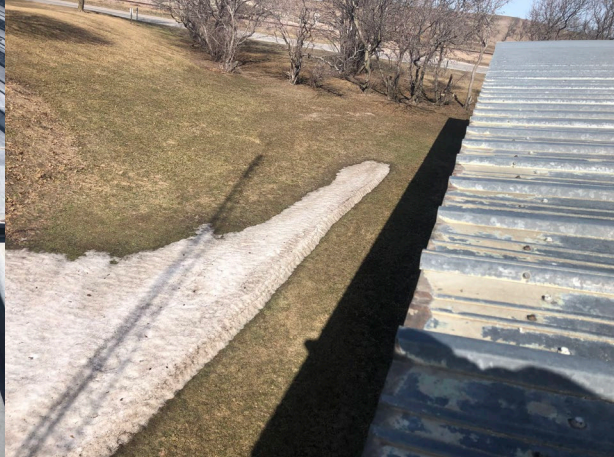
Missing gutters, evidence of rust beginning
