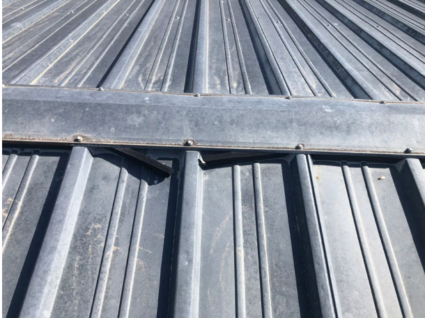
Deteriorated panel closures
