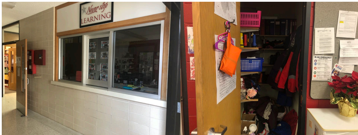
Reception desk is outside the entry vestibule Administration space lacks adequate storage The desk height is too tall to meet ADA
