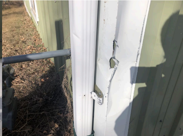
Damage to corner trim and downspout strap
