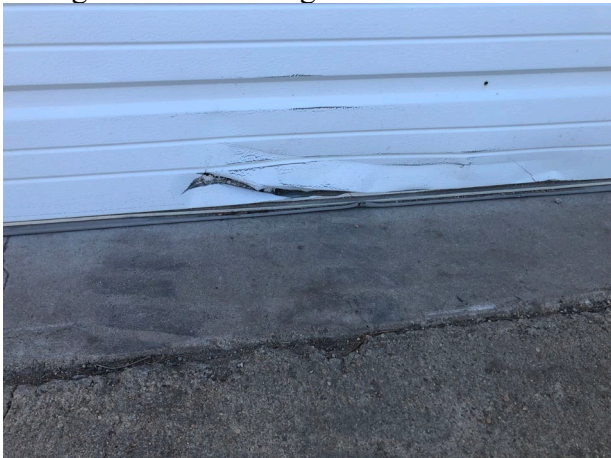
Overhead door damage
