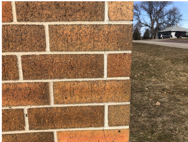
Crack in brick
