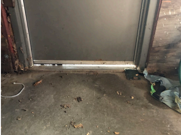
Walk door seals damaged
