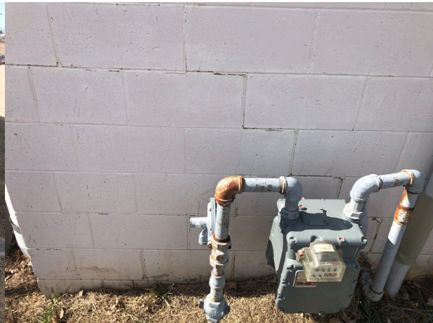
Typical mortar joint cracking in CMU
