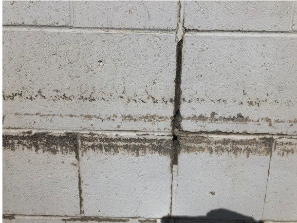
Soft joints in masonry deteriorating
