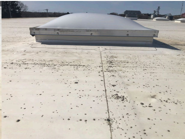
Algae should be removed to extend the life of the roofing
