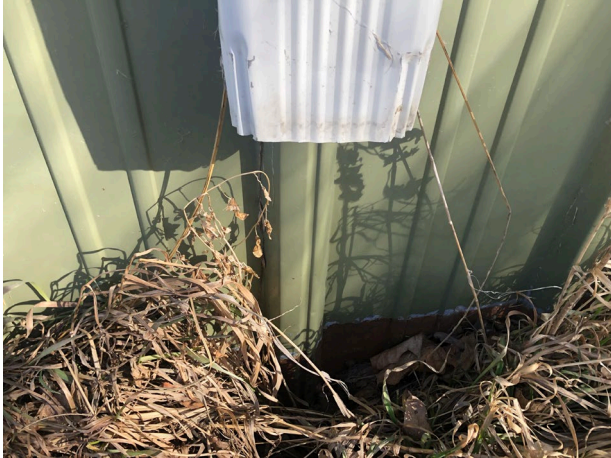
Missing splash block and downspout
