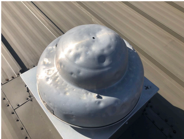
Hail damage to exhaust hood
