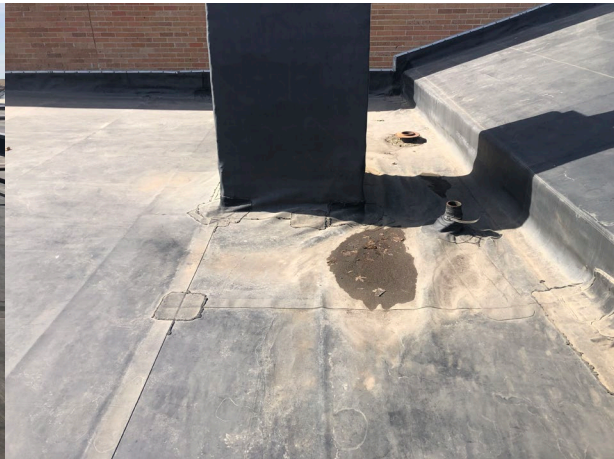
The roof deck around this chimney has completely rusted through. Standing water in this area is evident and was likely a contributing factor
