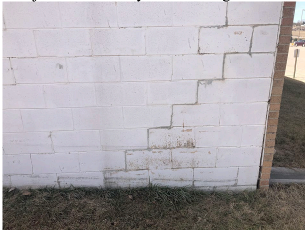
Typical mortar joint cracking in CMU
