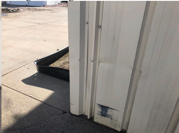
Typical siding damage
