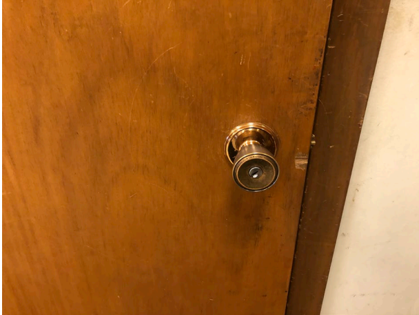
Interior hollow core residential door used for classroom door. Provides poor security and will not stand up to abuse. Note non ADA door hardware
