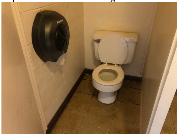
No grab bars, flush on wrong side, No maneuvering area, paper towel dispenser not in correct location
