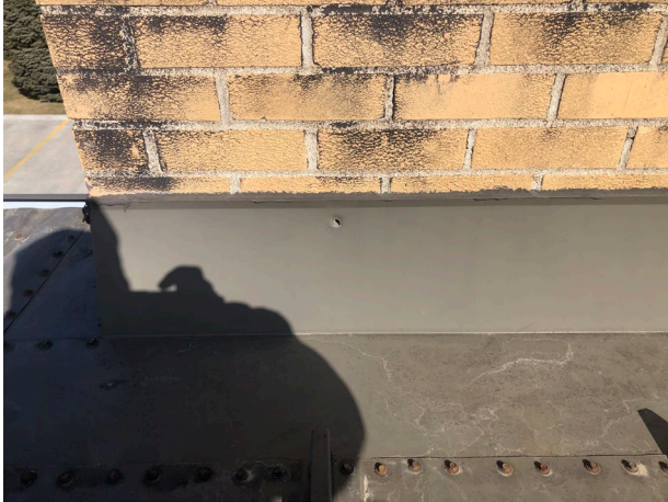
Missing fastener leaves hole in flashing
