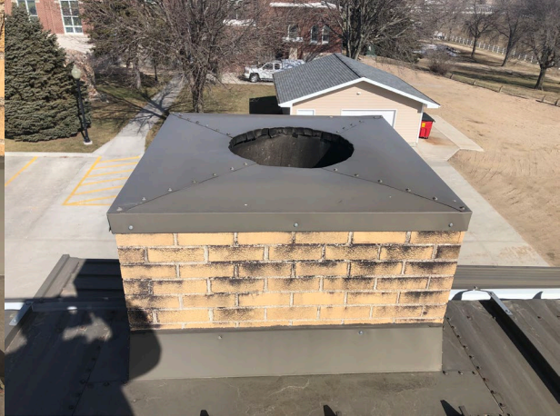
Chimney does not have a rain cap
