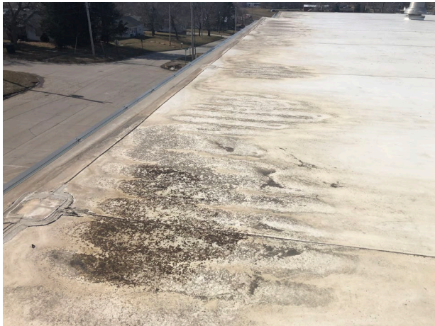
Fully adhered TPO / standing water should be eliminated
