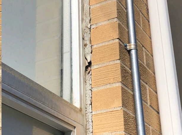
Deteriorating sealant at windows
