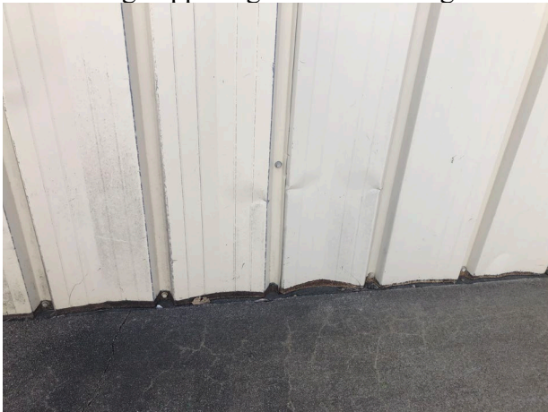
Typical siding damage
