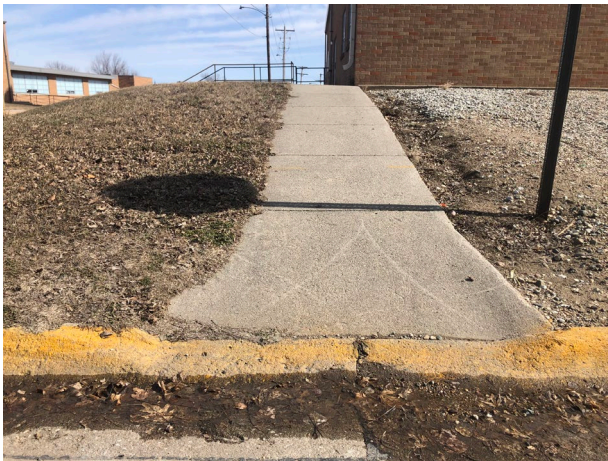
Non-compliant sidewalk and curb ramp
