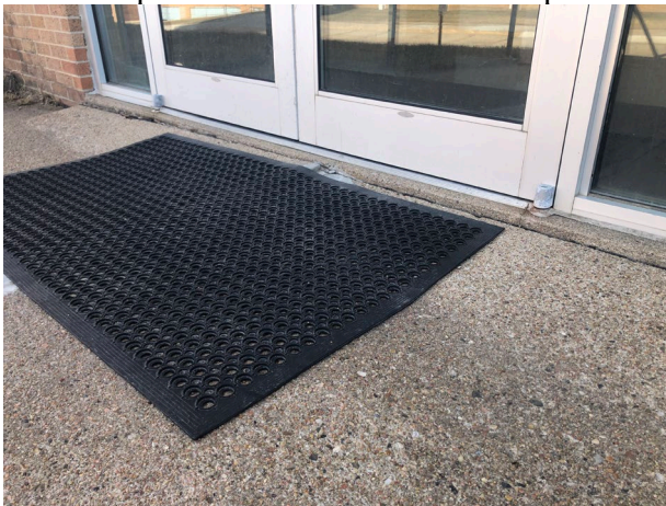
Vertical rise at entry door exceeds ADA
