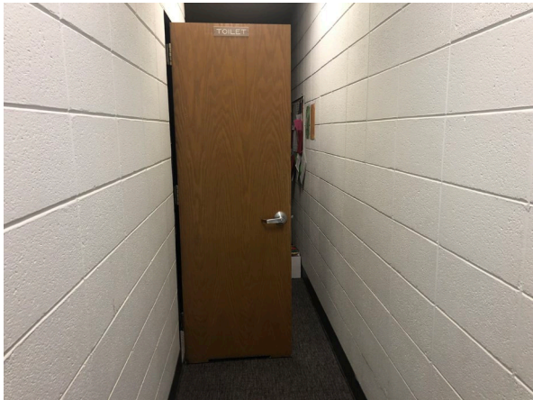
Maneuvering space at this door does not meet ADA
