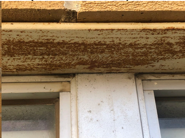
Steel window lintels starting to rust
