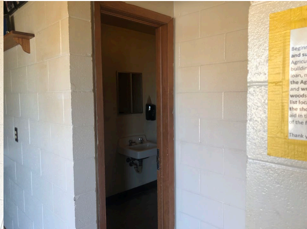
Restroom doors too narrow to allow wheelchairs
