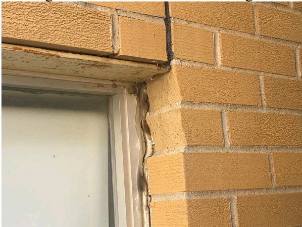
Broken bricks at window corners
