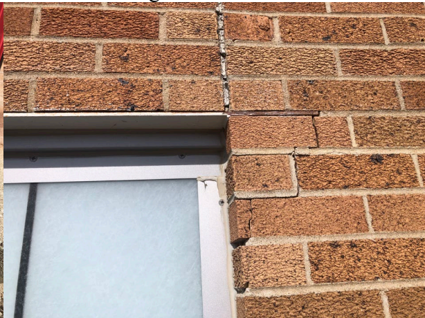
Control joint sealant has failed The steel lintel is rusting which leads to expansion and brick cracking
