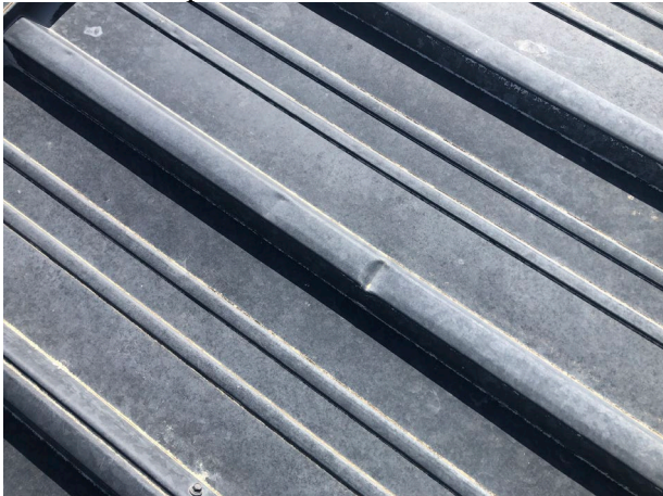
Finish gone, hail damage present
