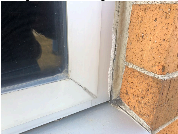
Sealant beginning to pull away from window
