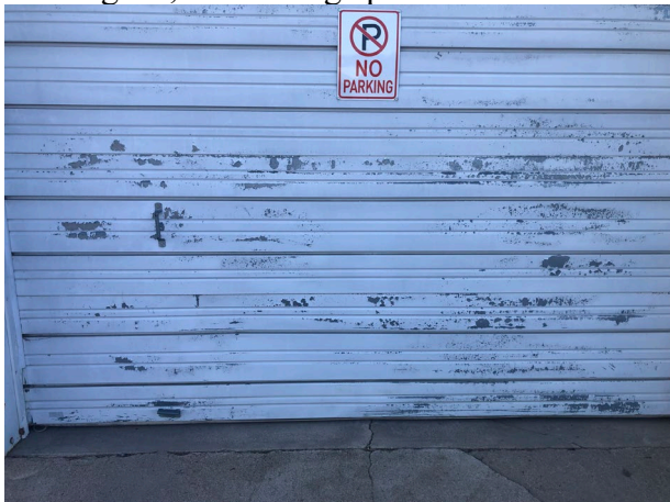
Damage to finish on overhead doors
